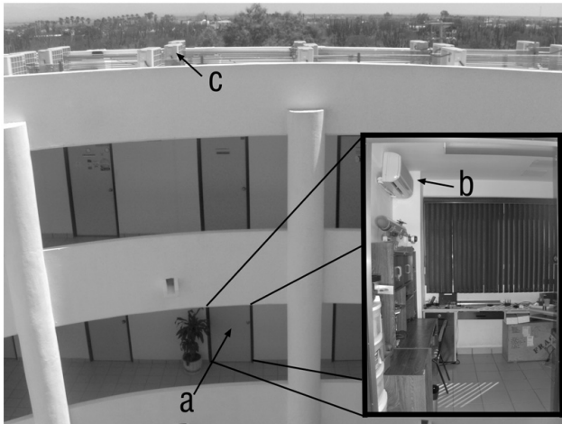
Figure 4. Experimental facility: a) office location, b) minisplit in office interior, and c) minisplit compressor.
